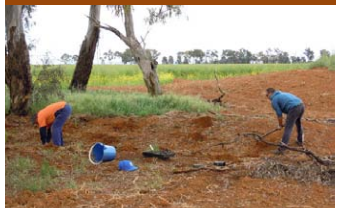
Wetlands are progressing. The wetlands are being developed with local community groups to demonstrate the 'green' aspects of agriculture and links with native ecosystems and biodiversity. The surrounding area was planted with native shrubs and grasses, in partnership with local aboriginal groups. Photo: Patricia Murray.
